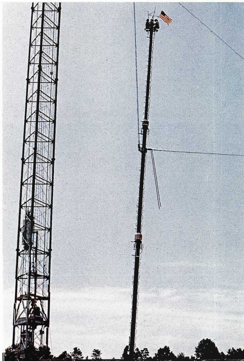
Trio of hardy riggers rest atop the TCL-16A Antenna as it leaves the ground.
