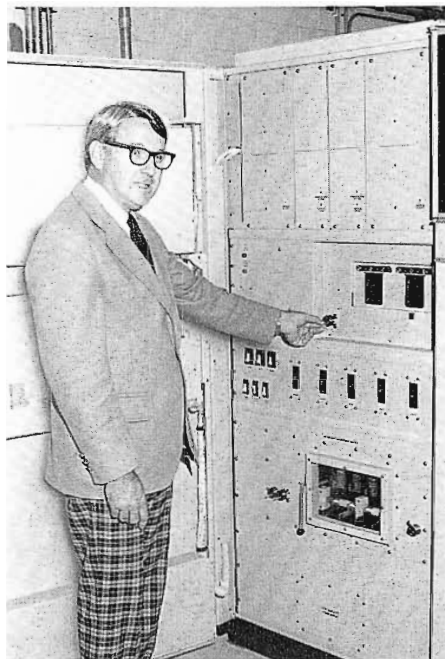
Bernie Moore, Vice President, Engineering at power supply cabinet of TTG-30/30H Transmitter. The key interlock system of TTG Series transmitters is an important safety feature for unattended operations such as that at WBTW-TV.
